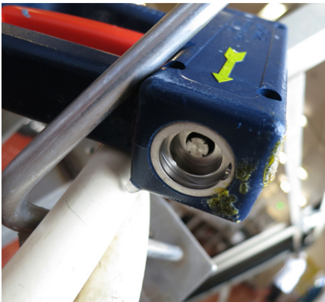
Installing flow restrictors in spray nozzles can conserve water and natural gas (used to heat the water).
