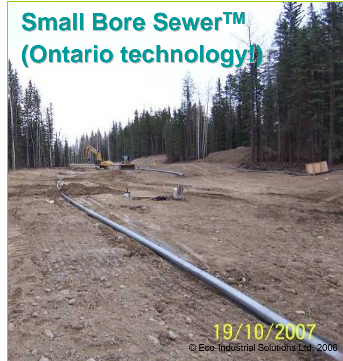
Small Bore Sewer™ (Ontario technology!) 19/10/2007 © Eco-Industrial Solutions Ltd, 2006 Installing new sewer Innovista Industrial Park Hinton, AB www.eip.hinton.ca
